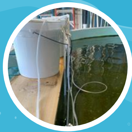
Air Pump System
